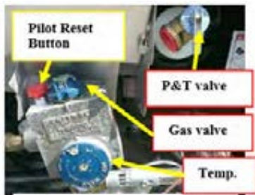
Water Heater pilot ignition
